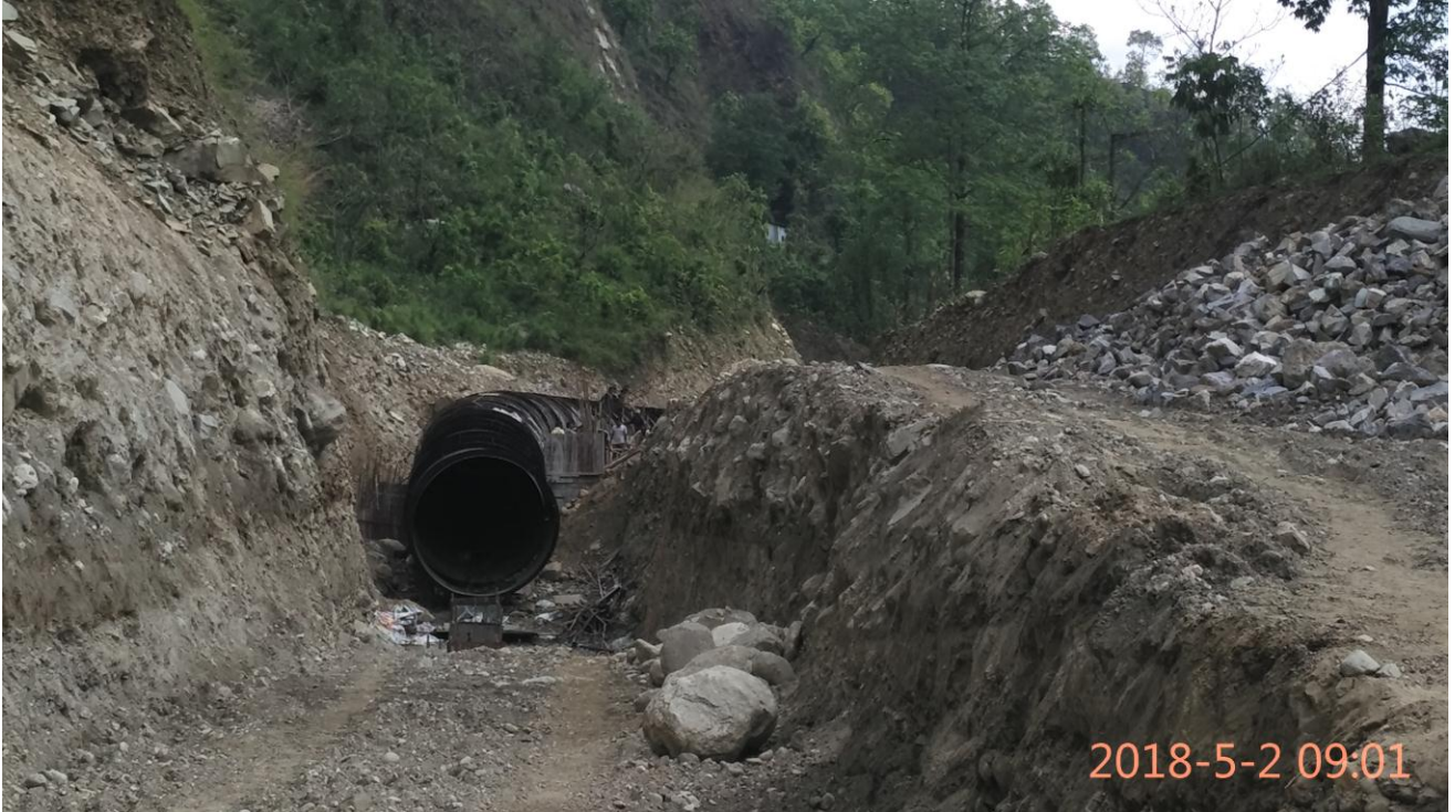
Penstock From D/S From CAB-4
